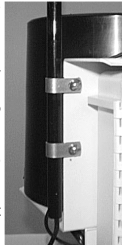
Anemometer clamped to back plate (unpainted clamps substituted for visibility)
